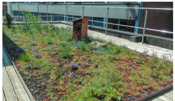
Blue green roof, Antwerp Photo: Vegetal ID
